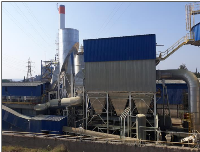
View of the plant
