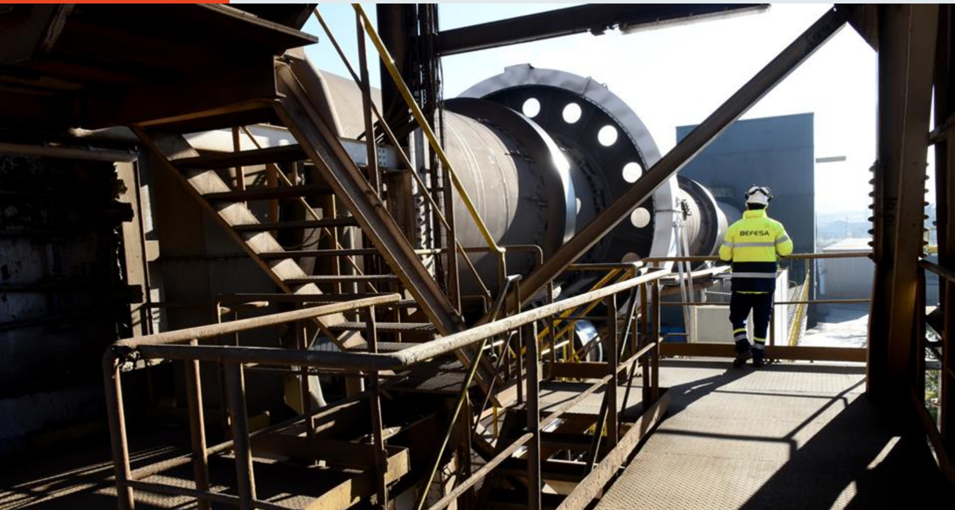
Electric arc furnace steel dust (EAFD) recycling plant at Asúa-Erandio, Spain
